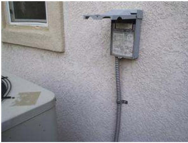
10.5 Picture 1 circuit breaker
