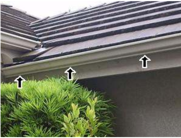
5.3 Picture 1 sagging gutter
