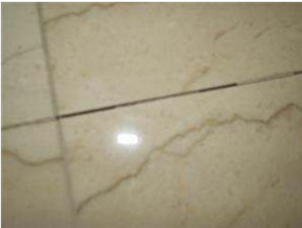
9.2 Picture 1 missing grout
